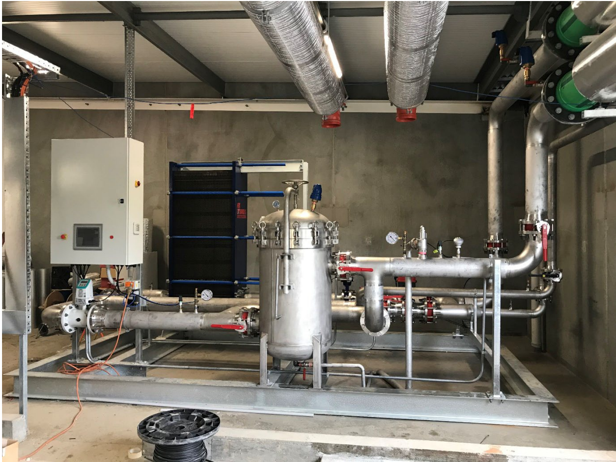
Figure 7.4 Geothermal heating system plant room at the Gippsland Aquatic Centre, Victoria, Australia.
