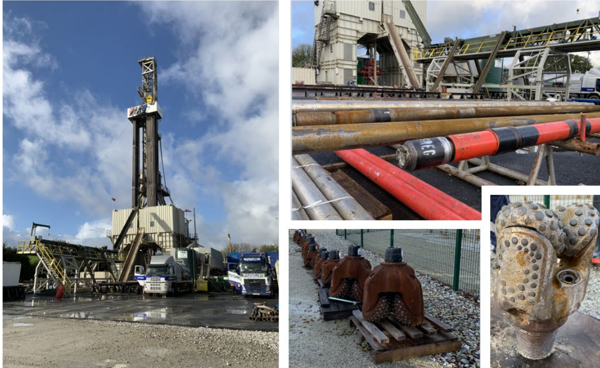
Figure 20.1 Drilling at Eden Geothermal Limited's site at the Eden Project in Cornwall (part funded by the European Regional Development Fund). Photo credit: Corinna Abesser
