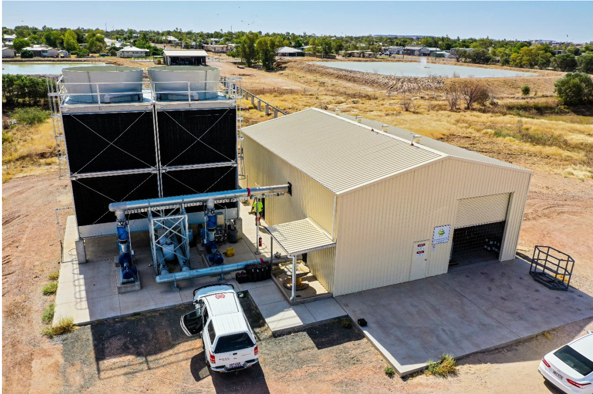
Figure 7.5 Winton Shire ORC geothermal plant.
