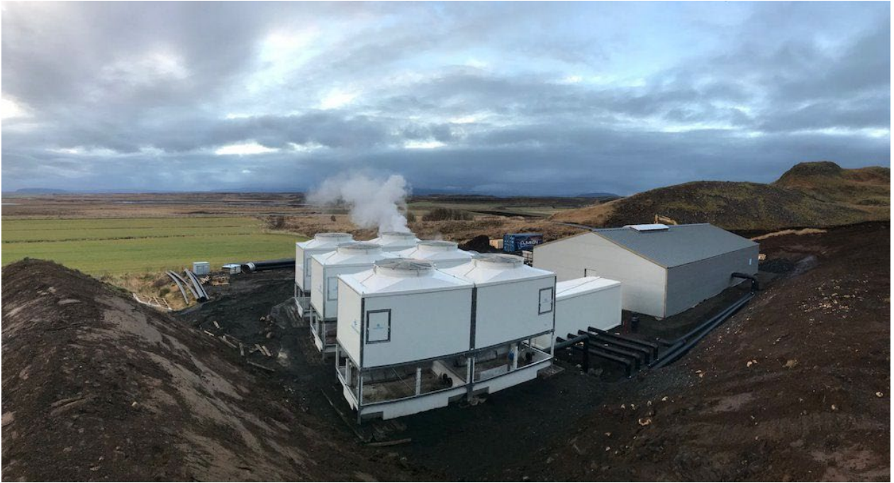
Figure 11.6. Electricity producing units by Climeon at the Flúðir field (Source: Climeon).
