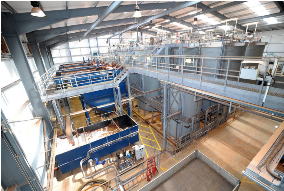
Figure 20.1 The Dawdon mine water treatment scheme that is being developed to supply mine water heating to a new housing complex in the northeast of England. Photo credit: The Coal Authority
