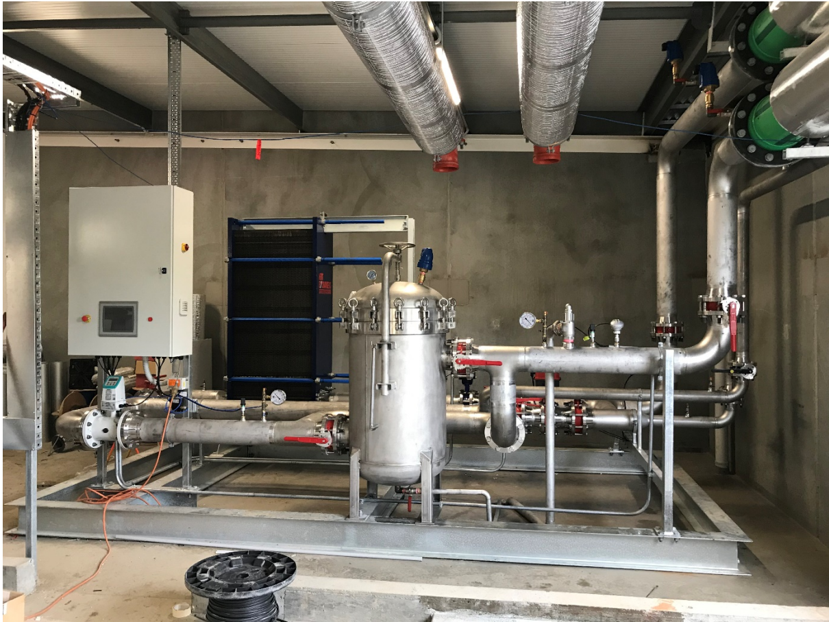
Figure 7.4 Geothermal heating system plant room at the Gippsland Aquatic Centre, Victoria, Australia.
