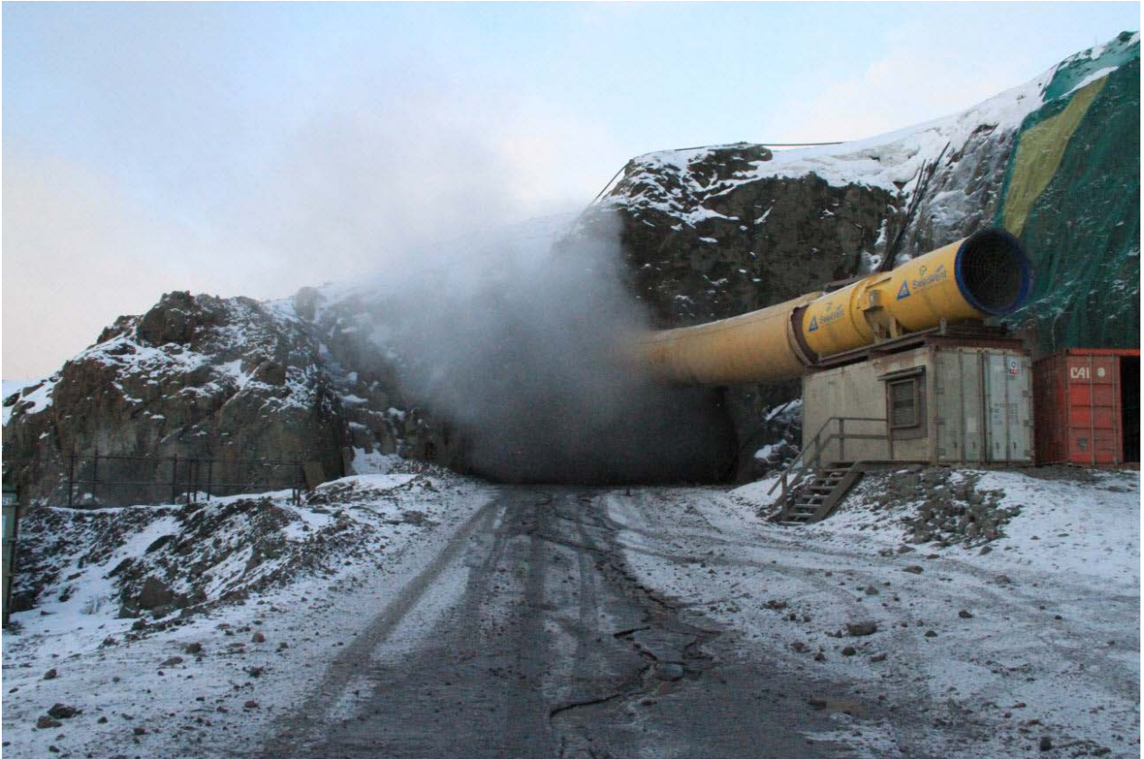
Figure 11.4. Hot water in the Vaðlaheiði tunnel in 2014 (Source: Vaðlaheiðargöng)
