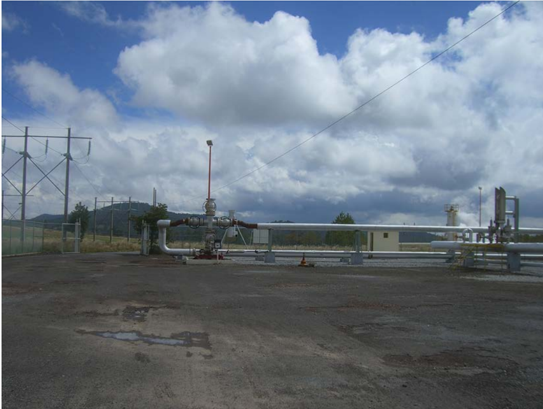
Figure 14.1 Los Humeros geothermal field (photo courtesy of CFE).
