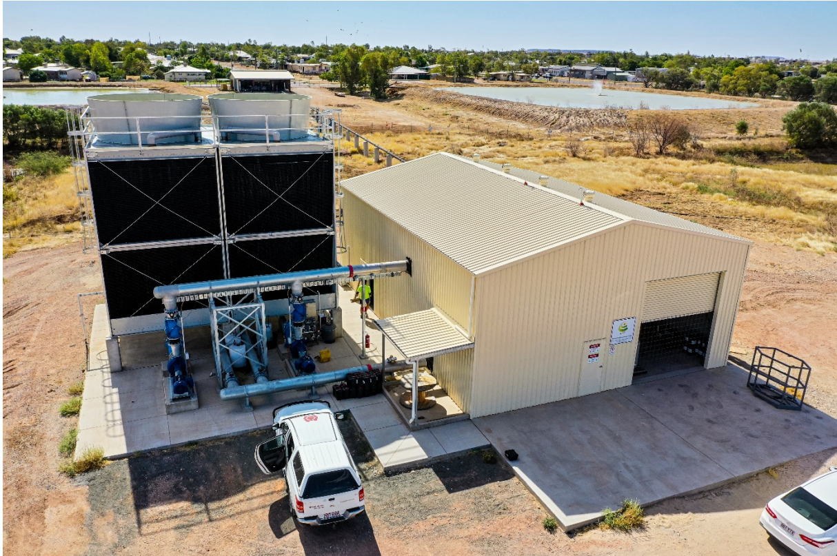
Figure 7.5 Winton Shire ORC geothermal plant.
