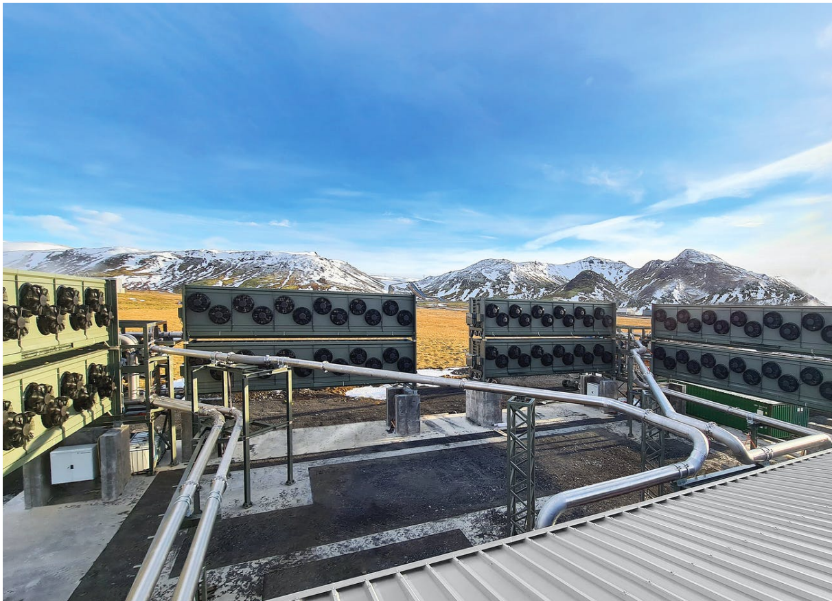
Figure 11.9. Climeworks CO 2 collectors at Hellisheiði power plant (Source: Climeworks).
