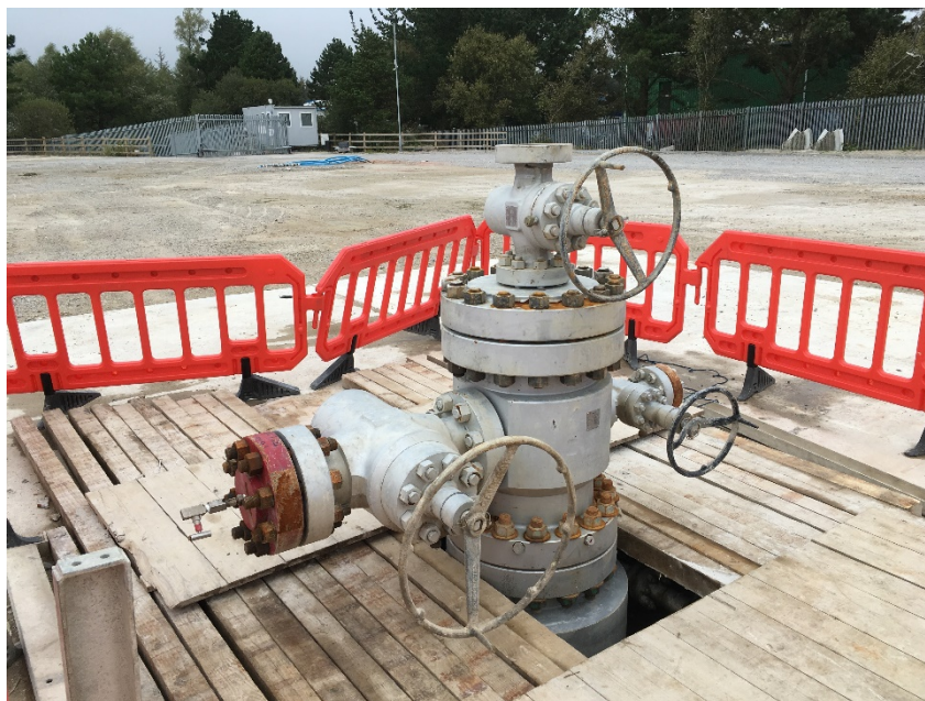
Figure 20-1 The UD1 well head at the United Downs Deep Geothermal Power project in Cornwall. Photo credit: Chris Rochelle, British Geological Survey
