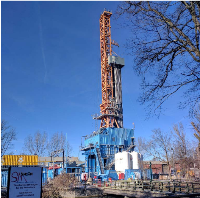
Figure 10-1 SWM Schäftlarnstraße geothermal project – Six wells drilled from April 2018 to the end of 2019
