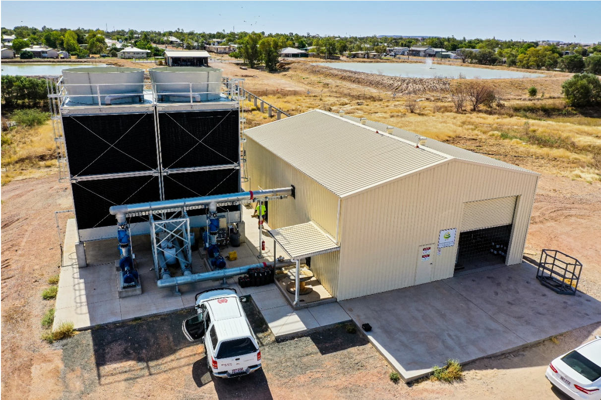
Figure 7-2 Winton Shire ORC geothermal plant.
