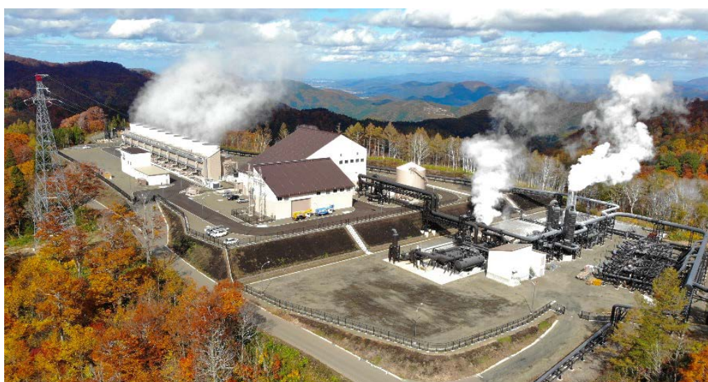
Figure 13-5 Wasabizawa Geothermal Power Plant (46,199 kW, double flush, since 20 May 2019). Photo by Yuzawa Geothermal Power Co., Ltd
