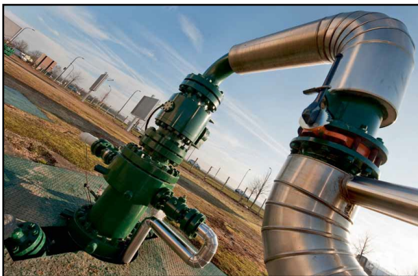
Figure 6: Well head of the Dogger geothermal plant in Melun l'Almont (ADEME)
