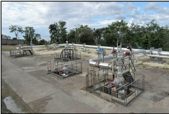
Figure 1: View of production wells of the Bouillante geothermal plant, (CFG Services)
