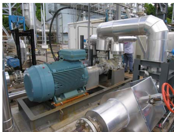
Figure1: View of Bouillante reinjection: a partial reinjection has been put in place to maintain the pressure in the reservoir. ©CFG Services - Géothermie Bouillante
