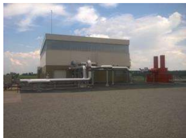
Figure 14: The Rittershoffen geothermal heat plant (source: ECOGI)
